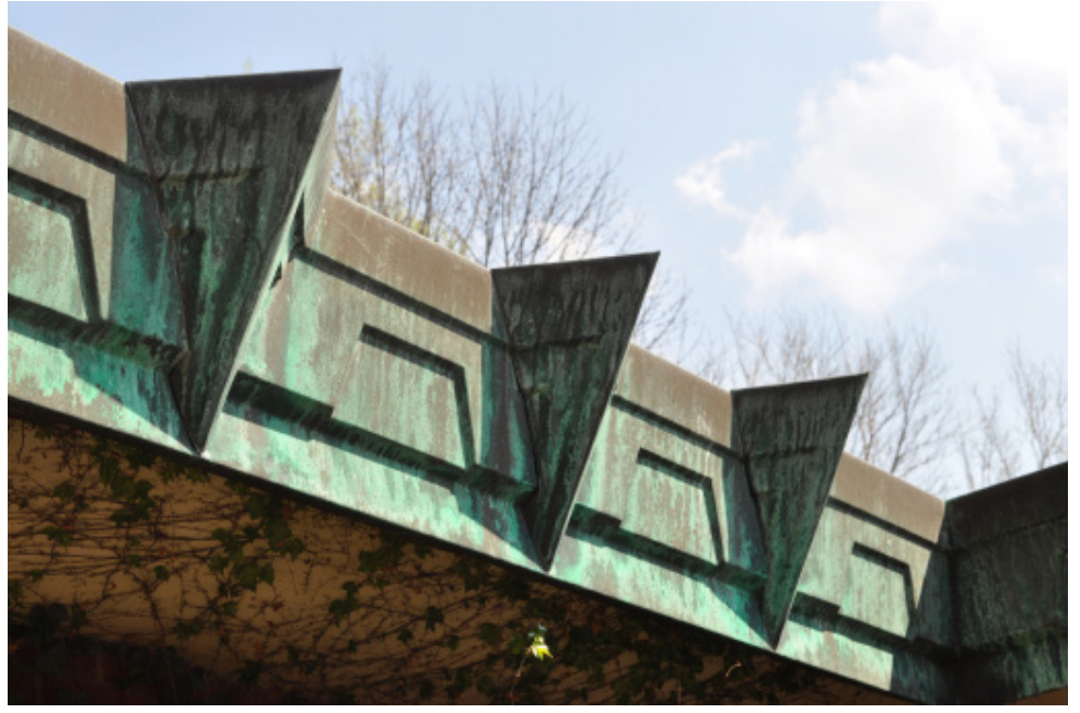
Samara, exterior, detail of roof with patinated copper fascia, 2012, digital image. Image: April Befort.
