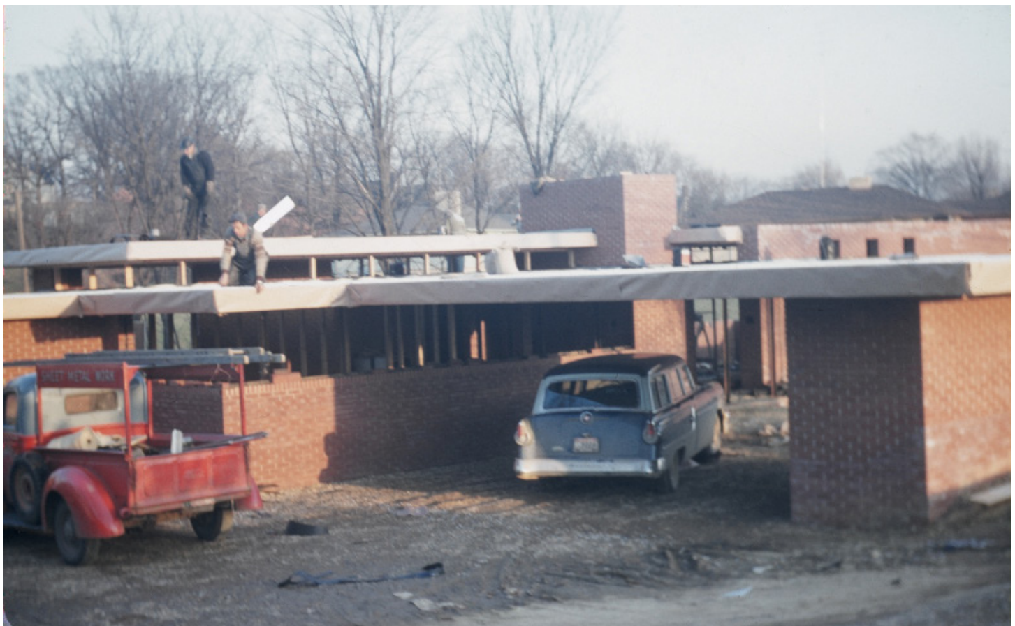
Samara under construction, exterior view of from driveway, 1950s, digital image of color photograph from Christian family album, courtesy John E. Christian Family Memorial Trust, Inc., West Lafayette, IN.
